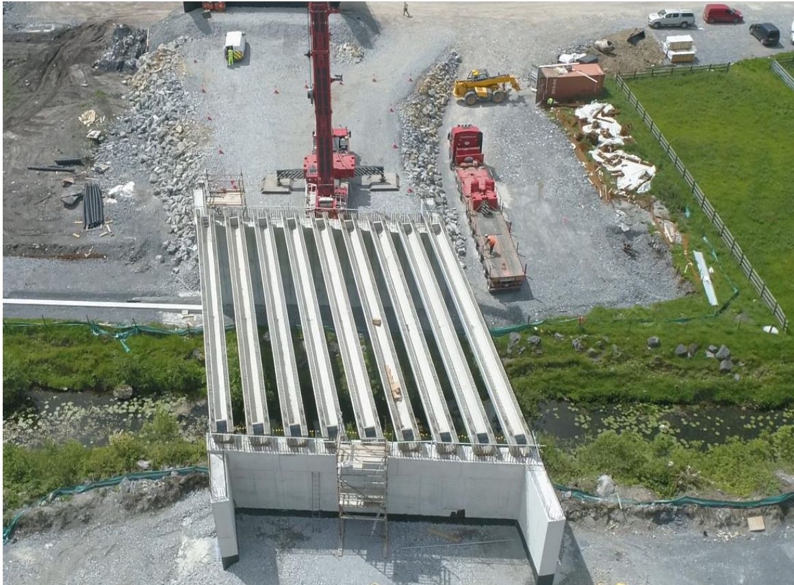
Installation of Pre-Cast Concrete Beams to ST04 – Bridge crossing over Ballyquirke canal
