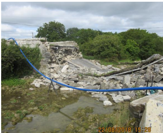
Dunkellin Bridge collapse August 2018
