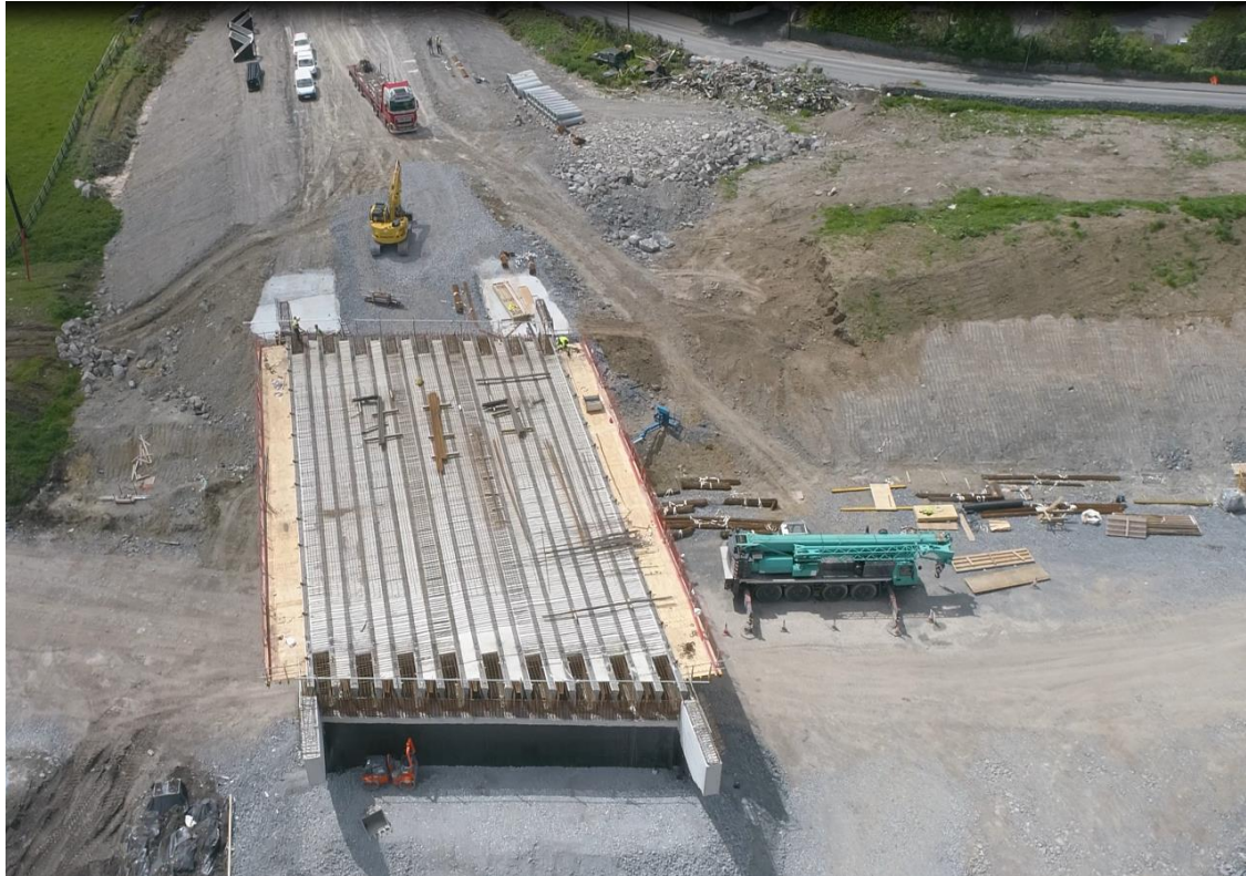
Preparation Works in progress for Deck of ST03 – New realigned Knockferry Road
