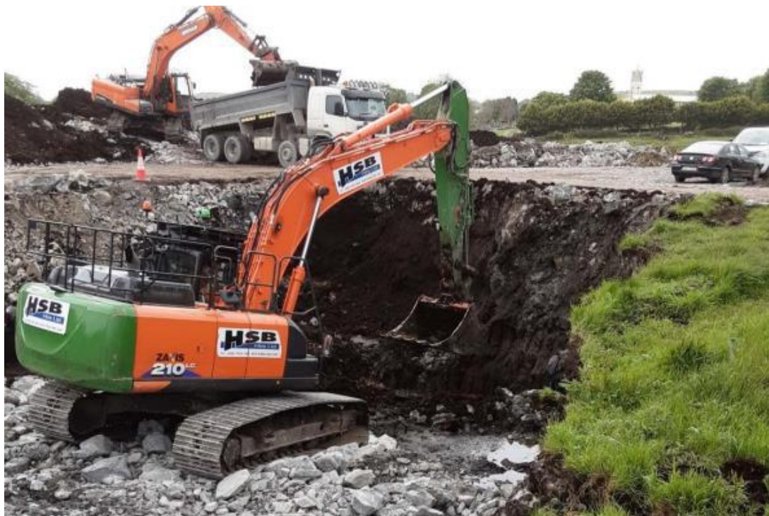
Earthworks excavation adjacent to the Homefarm Road – Note poor ground conditions and depth of excavation required
