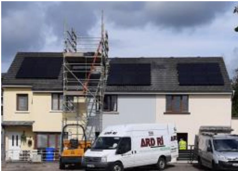
A Gort Mhaoilir, Athenry - 26 properties completed last week. Provisional BER Rating – A.
